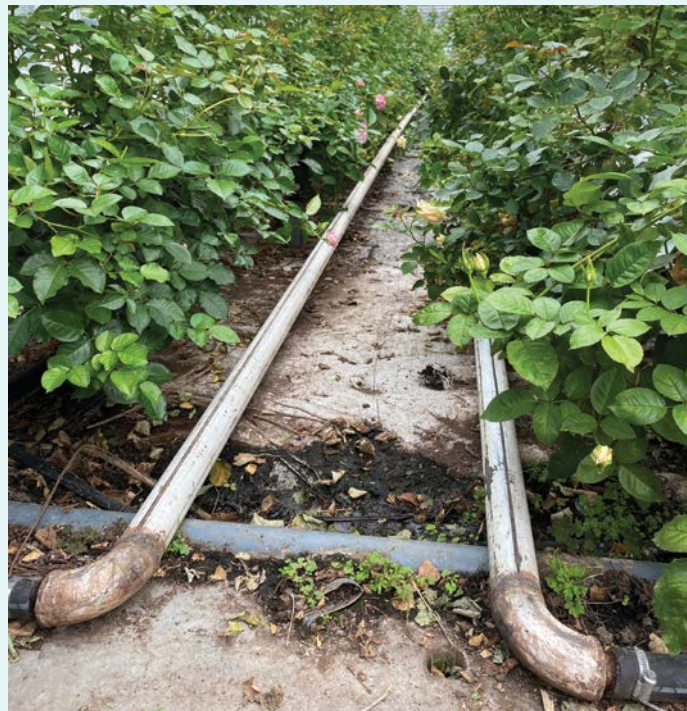
Pipes bring heat into the greenhouses
